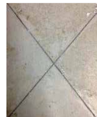
Paint applied to bare aluminum surface has completely delaminated
